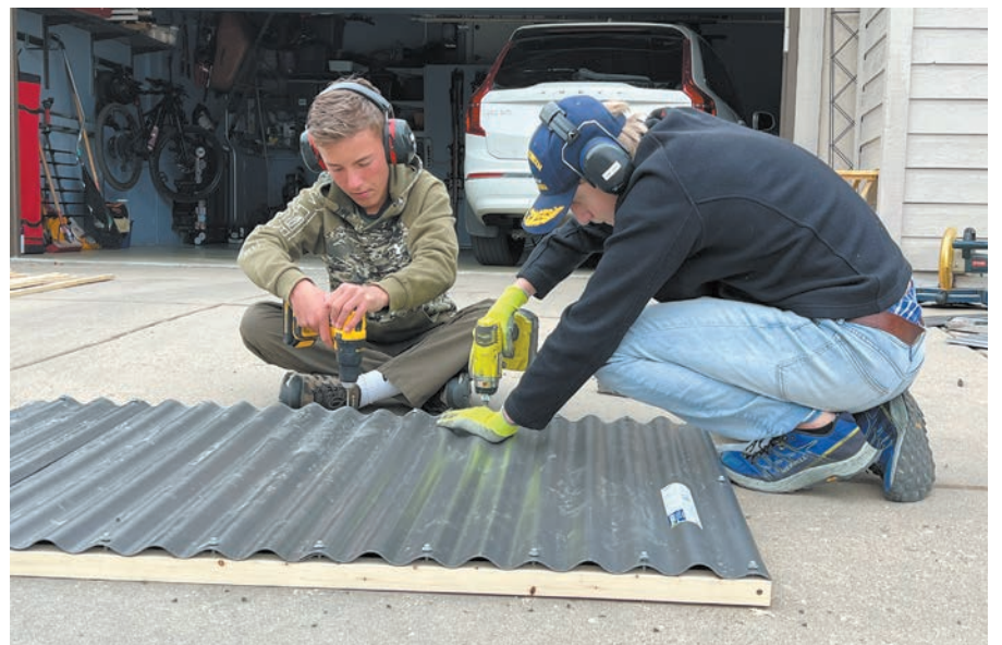
Conor and friend Kirwin Prendergast work to construct a roof of one of the five compost bins he designed and constructed as part of his Eagle Scout community impact project.
